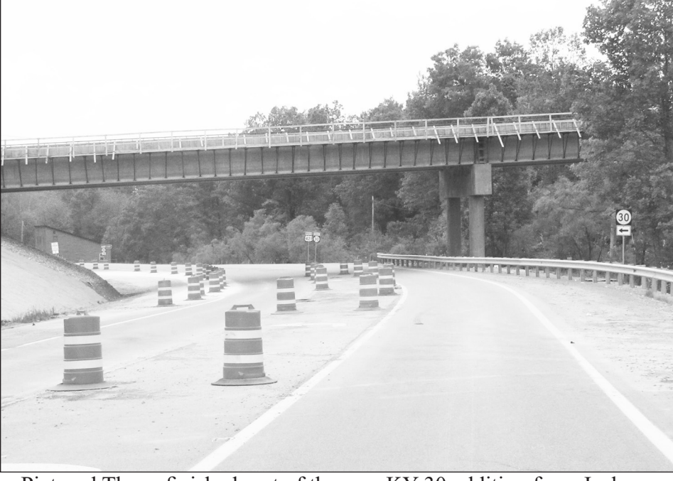
Pictured The unfinished part of the new KY 30 addition from Jackson County to Owsley County, which has work in progress at this time.
